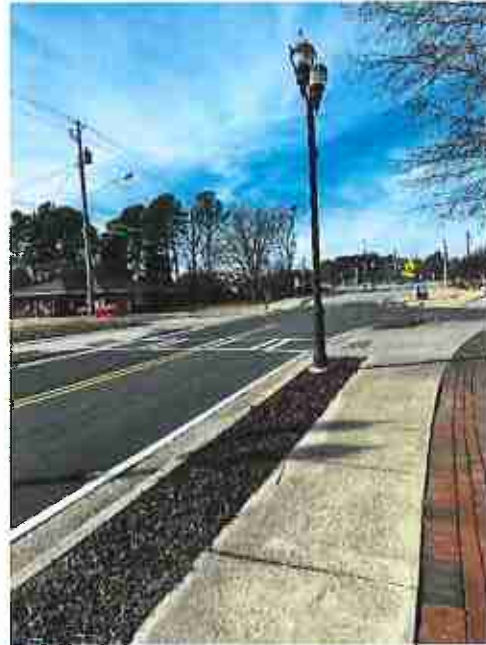
Lighting fixture in Green Zone
